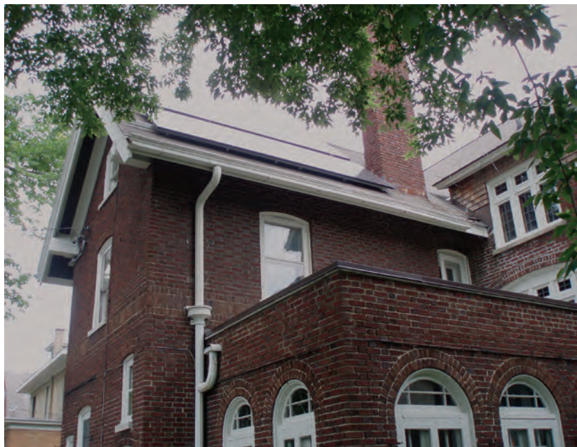
A PV system was installed on the rear elevation of this historic property in the Heritage Hill Historic District of Grand Rapids, Michigan. By locating the system in the rear of the property, the views from the public right-of-way remain preserved.
